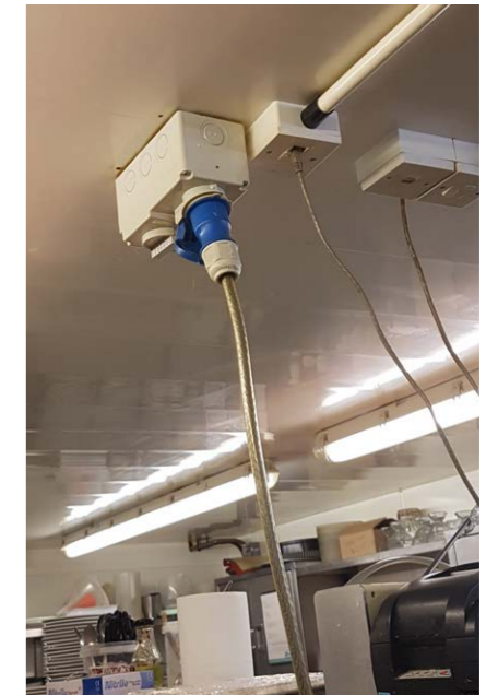
The electricity and gas supply are high up and can be easily turned off and back on.
