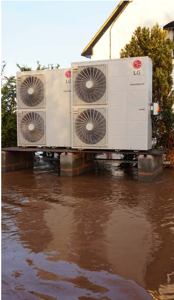
Air source heat pumps have been placed up away from flood risk.
