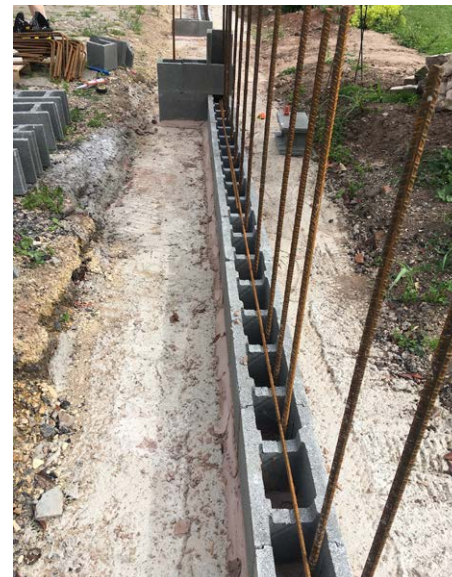
The pre-cut lengths of bars were placed in the groove in the block and tied to the vertical rebar
