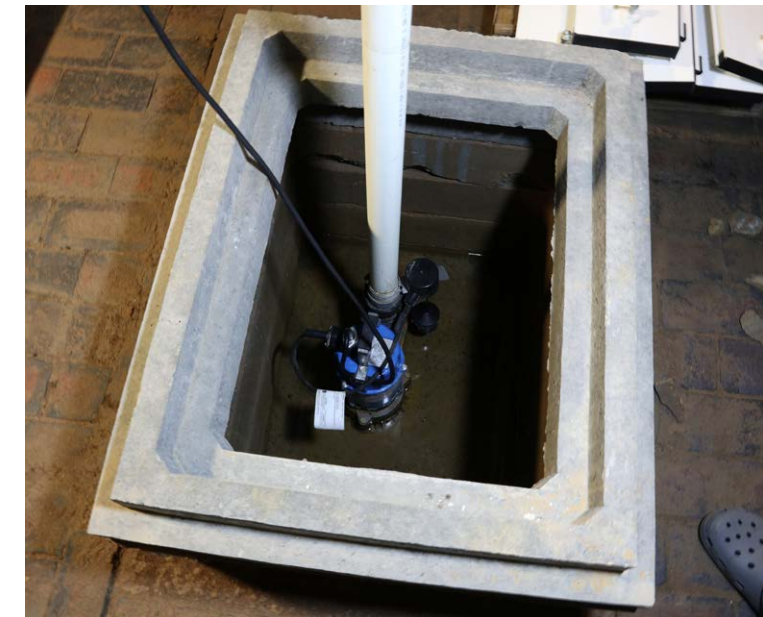
Two more pumps in the cellar.
