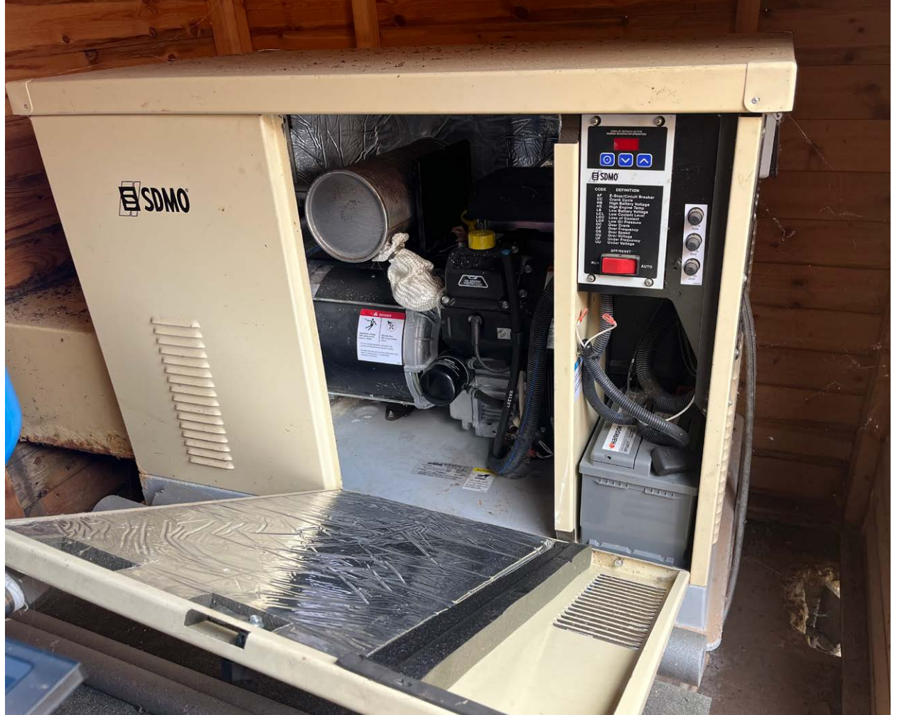
LPG Backup generator, strong enough to run the pumps during a power cut.
