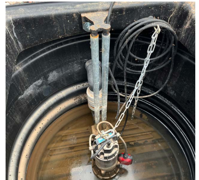
The sump has a rail system for easy replacement of a failed pump
