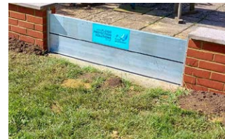
Flood Protection Solutions
