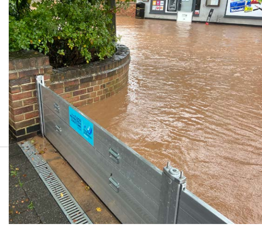
Flood Protection Solutions
