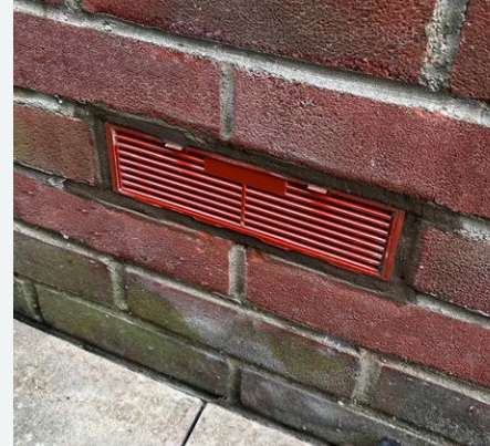
Buffalo Flood Systems
